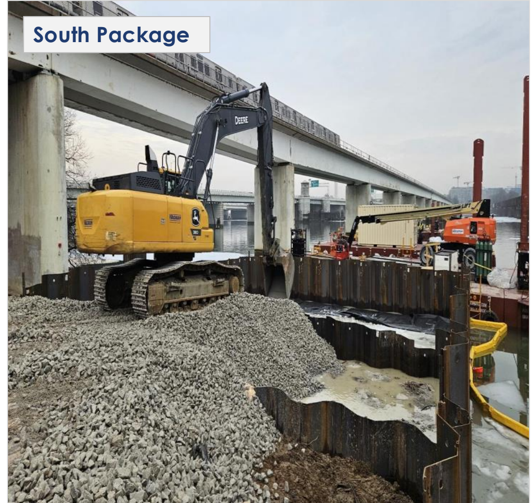
Crews are preparing access bulkheads on both shores of the river that will be used to launch construction equipment and materials onto barges.
