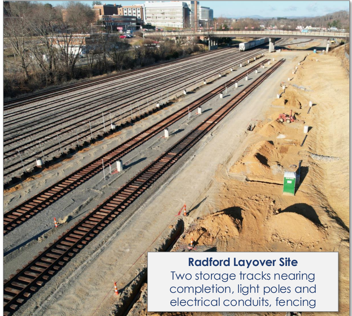
Cambria Station Site Platform construction, parking lot grading, retaining walls, station track and turnouts
