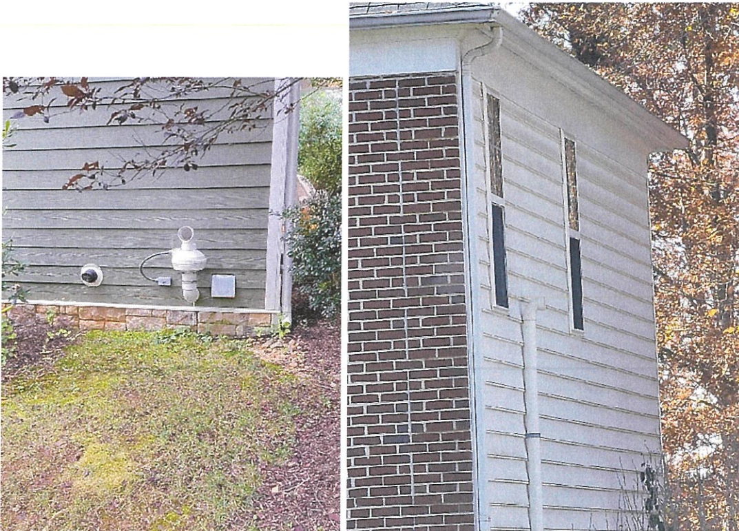
Charlottesville, VA - These we noticed on neighboring homes where we installed radon mitigation. You can drive around Glenmore, a gated community just outside Charlottesville and find many systems just exhausting within eight feet from ground level or just under or next to upper story bedroom windows.
