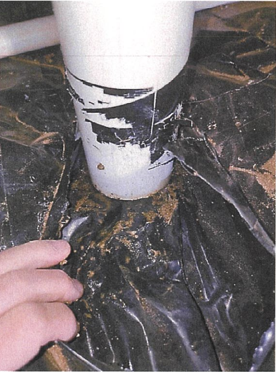
Rockville, VA – 2025 new home, builder of this development is telling buyers that all the homes have passive radon system. A couple of months ago the homeowner who is working from the home decided to purchase a home radon monitor. Levels were over the action limit. We were contacted to convert the ‘passive’ system to an ‘active’ system. Found the builders passive vent, installed the fan to find there is no
