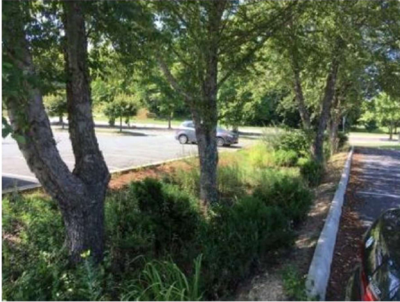
Figure P-FIL-05-12 An older bioretention area with mature tree growth and shaded areas. Adaptive management is required in areas such as these for continued performance.
