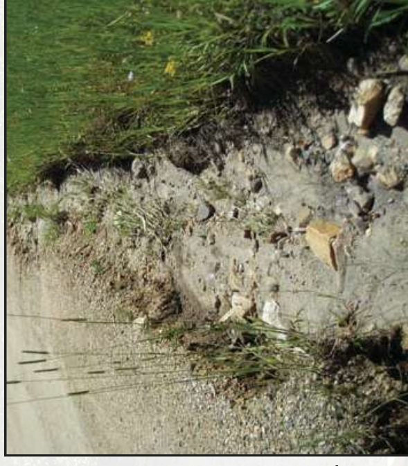
Figure 4.19—Unstable ditch. This ditch presents a safety, maintenance, and environmental concern. It is too deep, too wide, unvegetated, and can route sediment to the stream.
