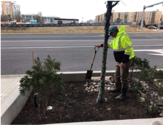
Figure P-FIL-05-5 Image of Ultra-urban bioretention/tree planter cell receiving curb/road drainage in Fairfax VA
