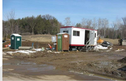
Example of Poorly Maintained Vehicular Route Stabilization
